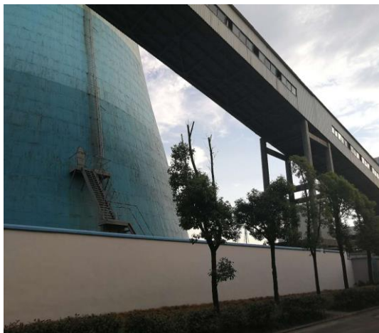
冷却塔隔音屏
